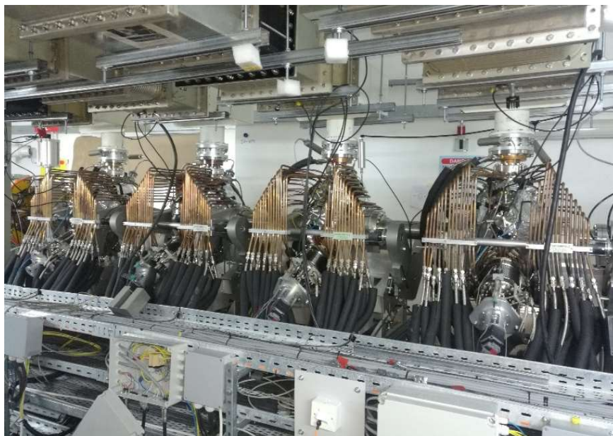
Four RF cavities in the SESAME storage ring
